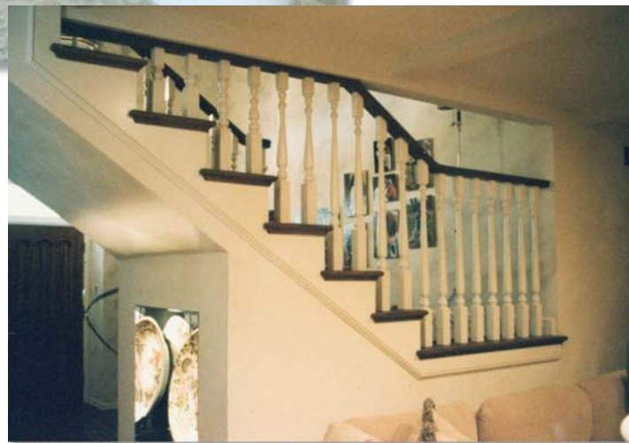
This awkward situation is caused by the upper floor overlapping the stair. The opening in the upper floor should be big enough to allow the rail to pass through.
